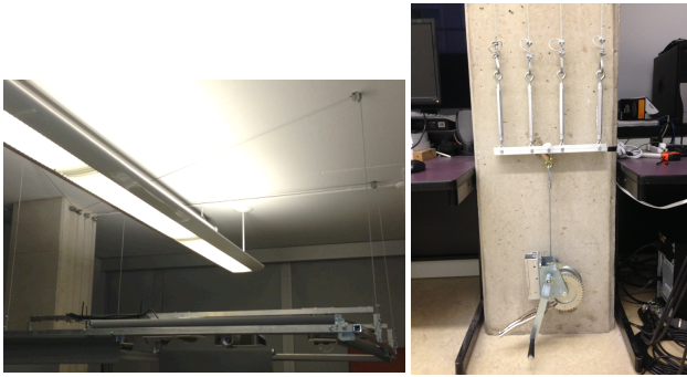
Figure 2: Cable system to support the frame, on which all system components are mounted. We created this for development convenience.
